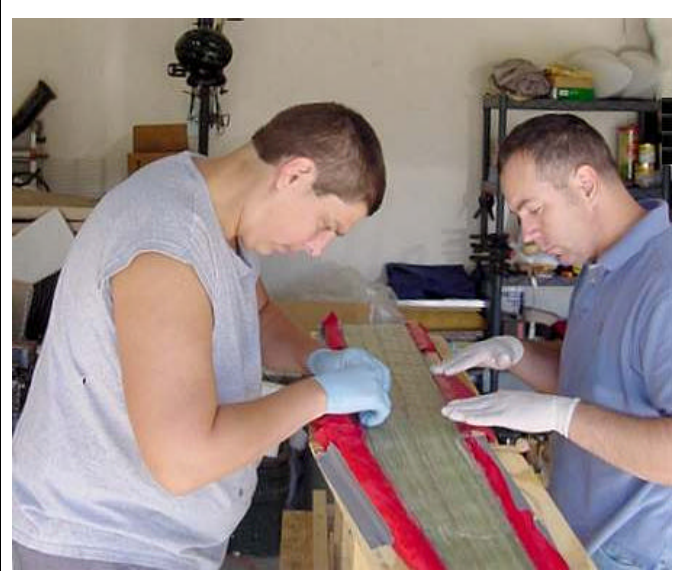
Jeff (right) and Drew (left) work at laying the glass in place
